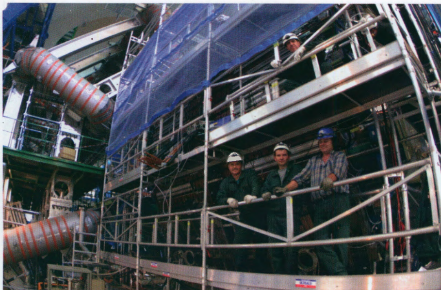
The ATLAS facility
