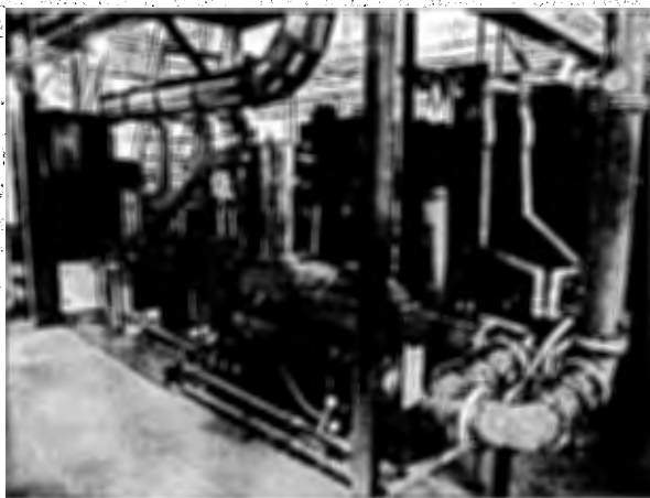
Fig. 1: New DFELL generator
