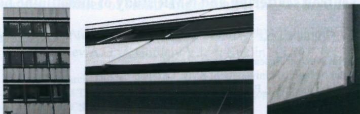
Fig. 2 Behavior of the marble panels on the economic building in Goettingen.
