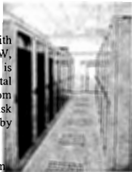
Fig. 1. The new computer room from 2004
